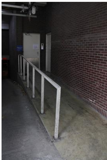
Hellingbaan in garage
